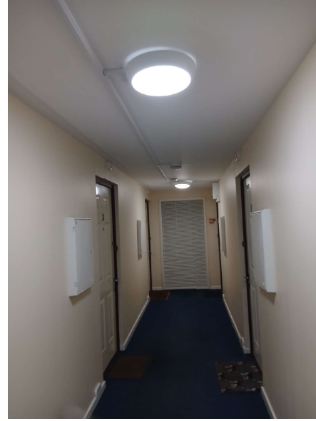
Lighting (Standard and Emergency Lights)
